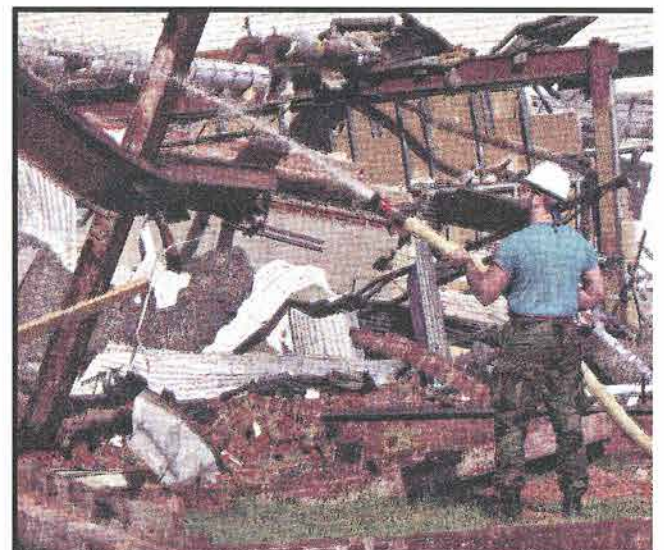
Paul Moldenhauer, a demolition worker, hoses down debris to minimize dust on the opening day of demolition at North Hills Mall. The job will take several months.
